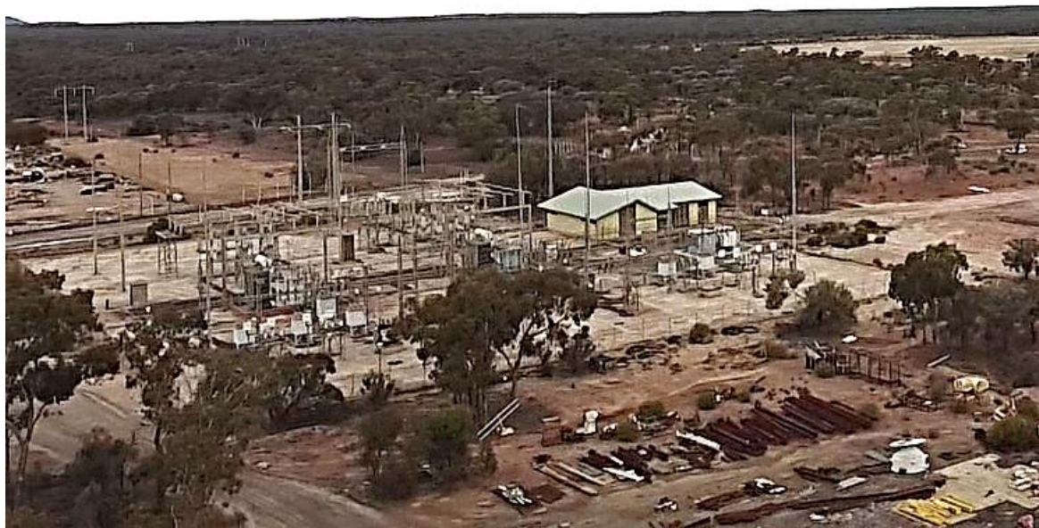
Figure 38: Electrical Sub Station on Site
