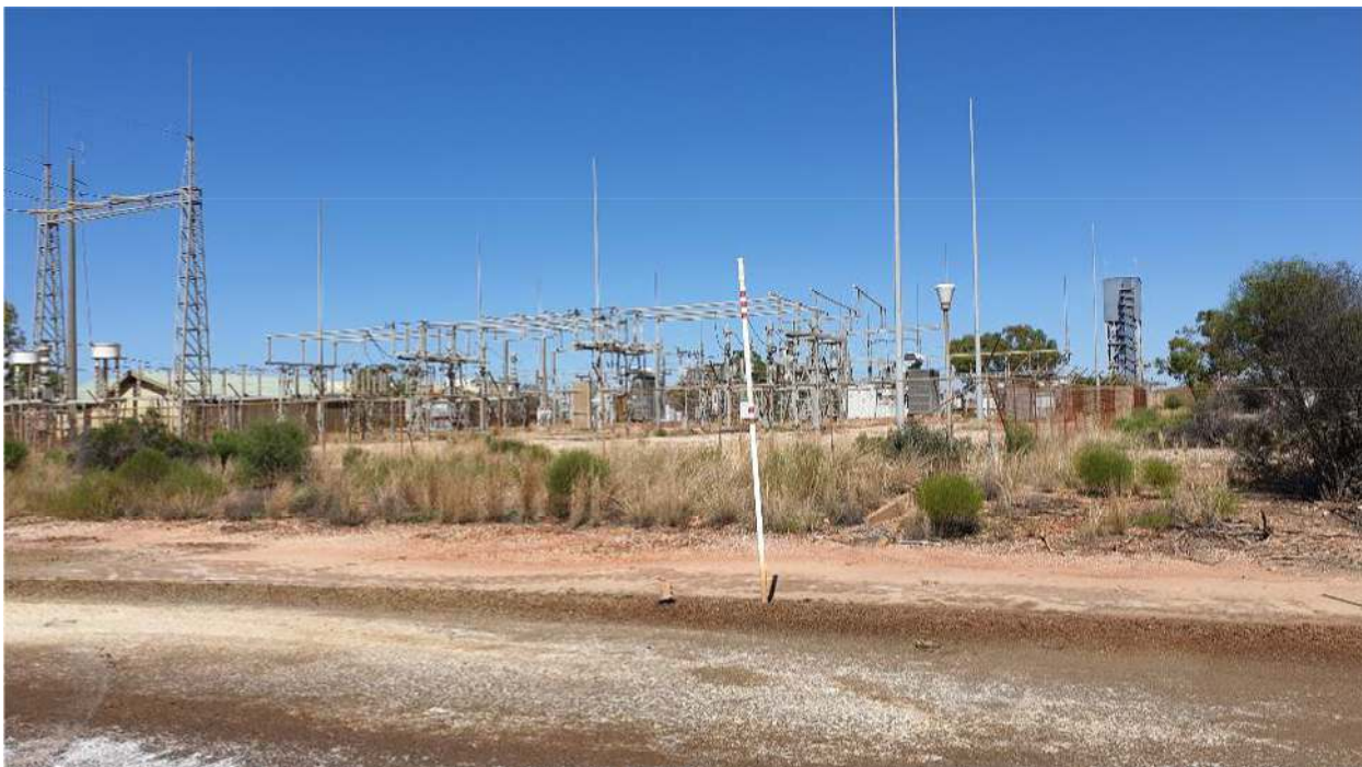
Photo 9 - Main Sub Station
