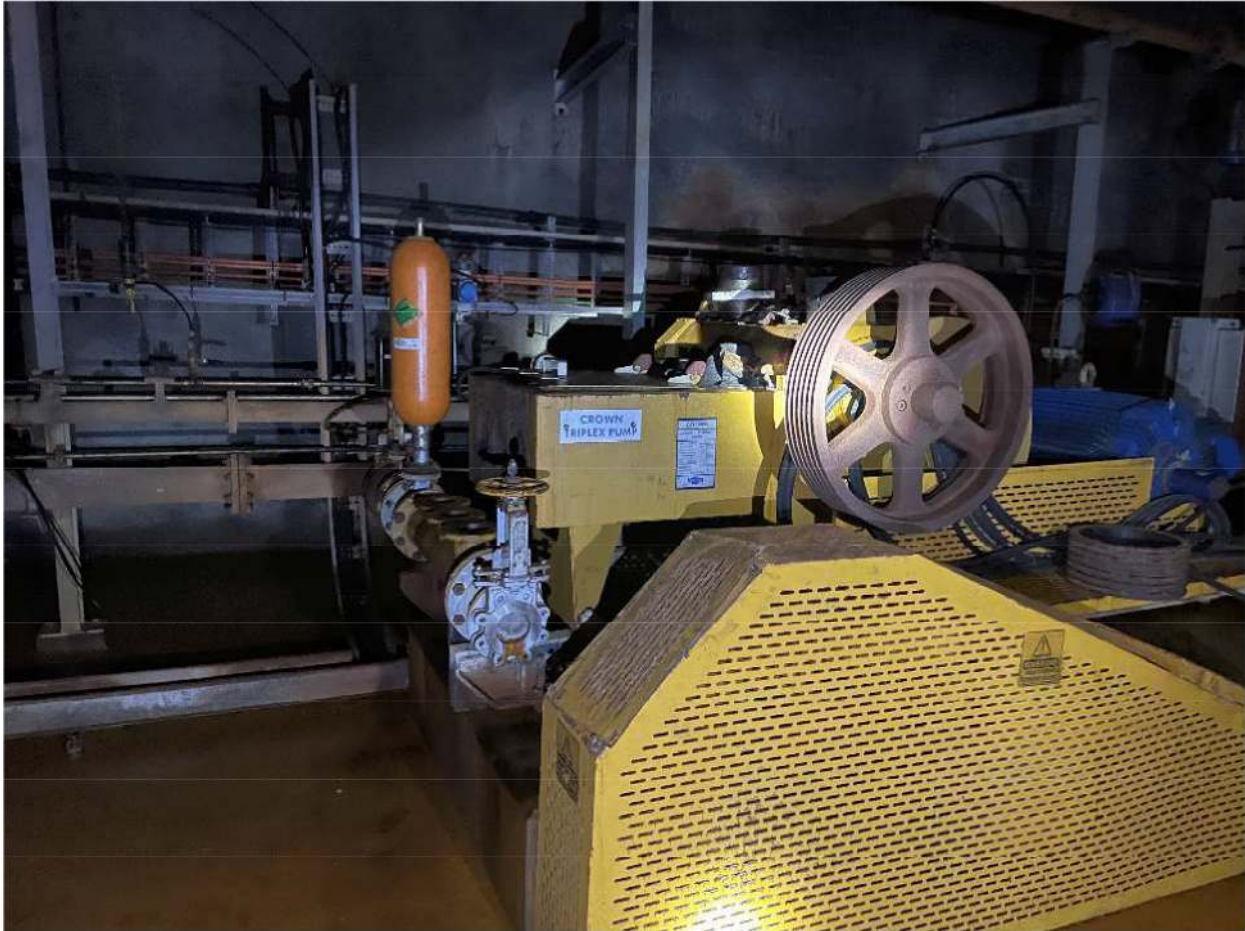
Photo 8 - 930m Pump Station
